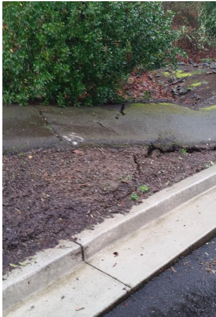
Detail view in west portion of landslide showing pavement cracks in asphalt sidewalk, tension cracks in unpaved dirt area, and joint opening between concrete curb and asphalt roadway.
