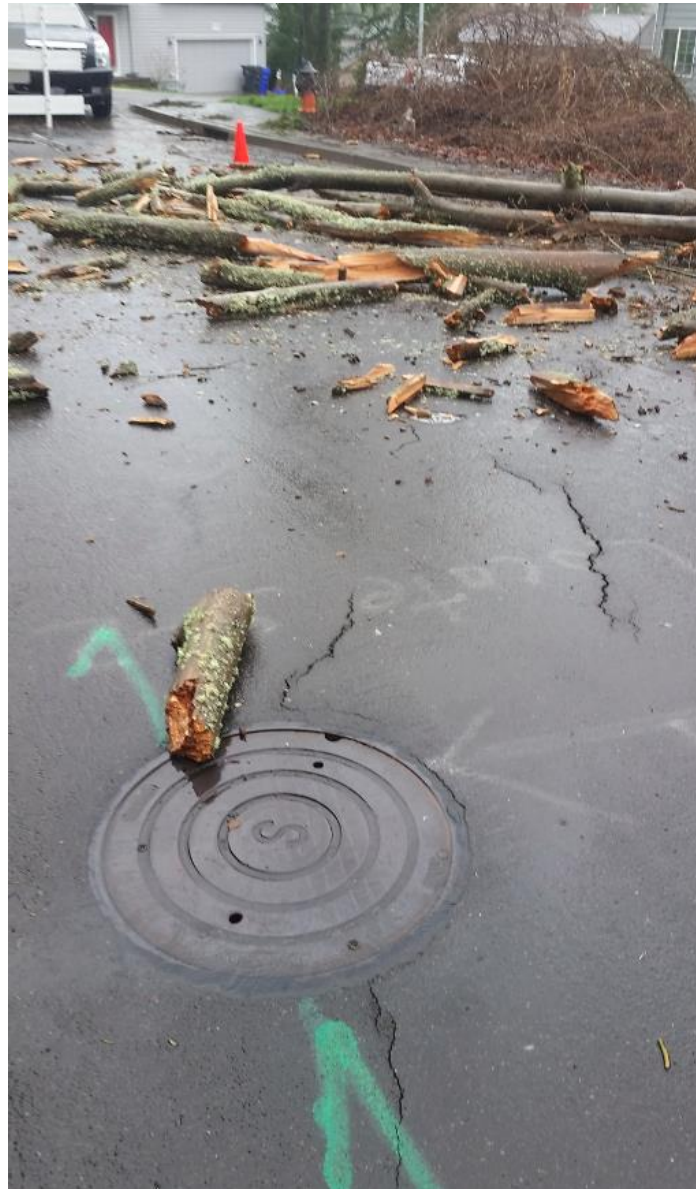
Detail view in north portion of landslide showing pavement cracks around sewer manhole.
