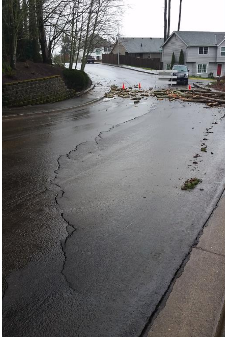
View north showing pavement cracks. Note downed tree pieces in background.
